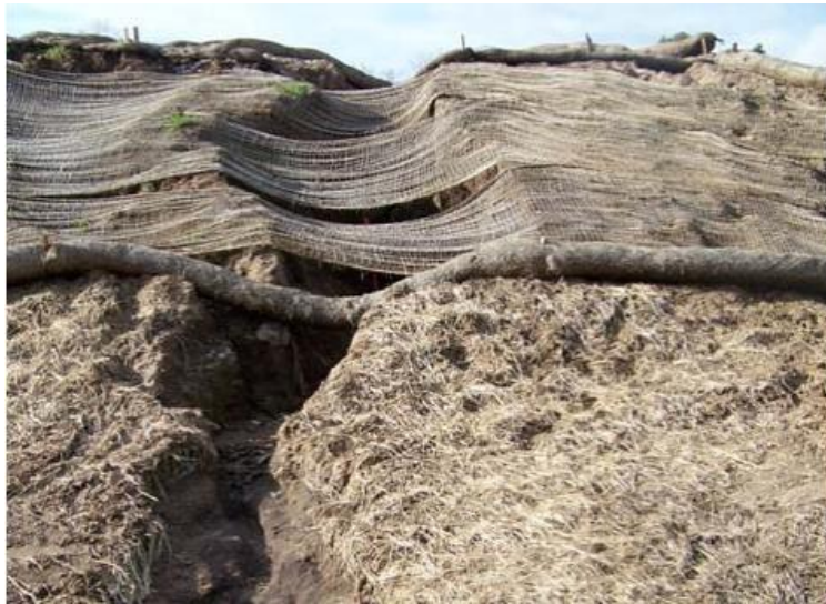
Figure 6-1 Erosion on fill-slope from concentrated flow.
