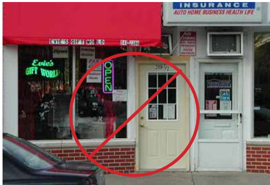
Prohibited: Residential Grade Doors on Commercial Buildings
