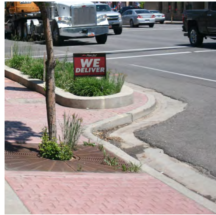
Fig 11: Existing Conditions - Deteriorated Curb and Gutter
