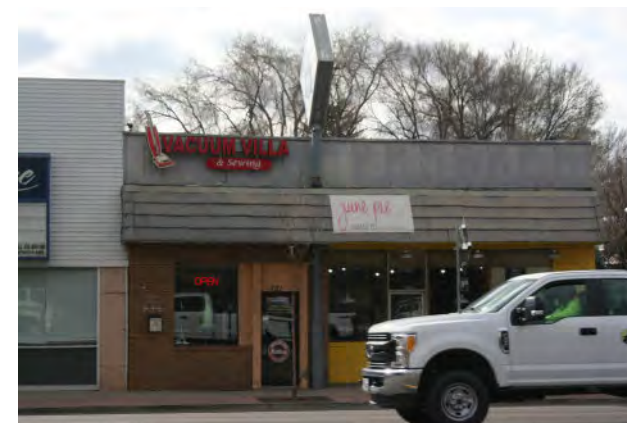
Fig 23: Existing Conditions - Deteriorated Façade
